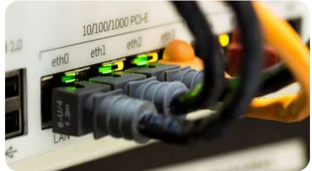
Switch, RAN and Router
