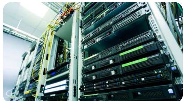
Rectifier, Battery and Server
